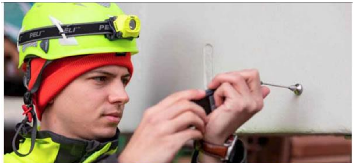
Beaux Ackx , Coating Inspector for SCICON worldwide checks the DFT of the first coat of Ecoshield
